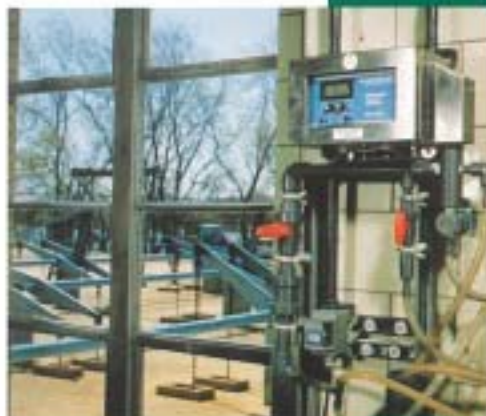
Municipal water treatment
