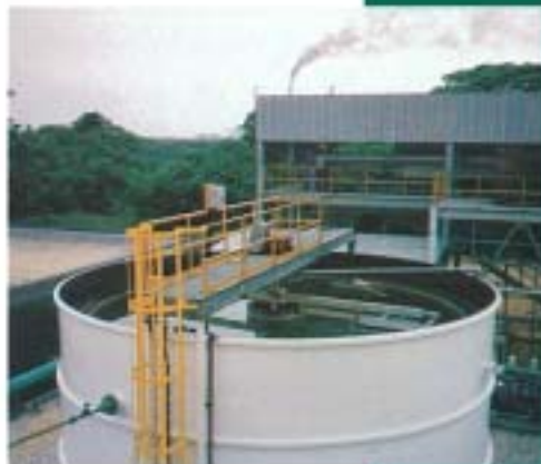
Municipal or industrial wastewater treatment
